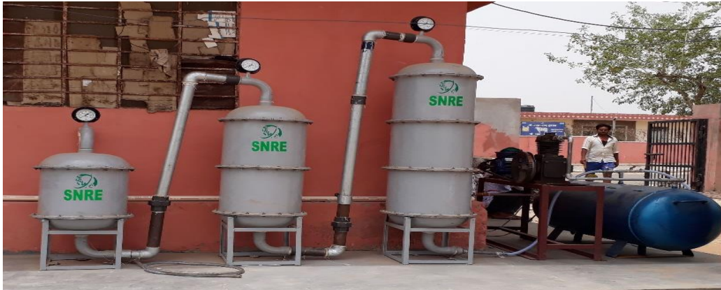
Scrubber installed based on PSA technology
