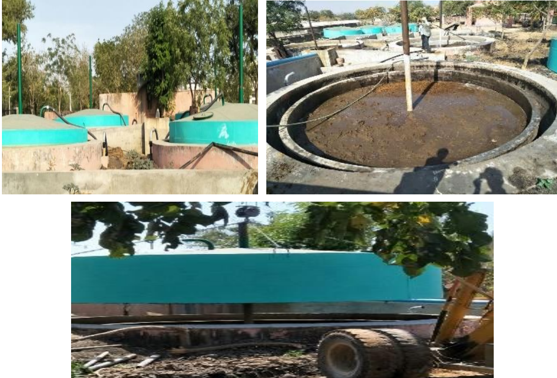
Picks of the Digester with dome over it with fitments
