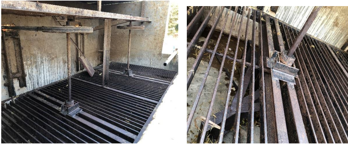
Picks of the missing pit with agitator placement and the metal platform
