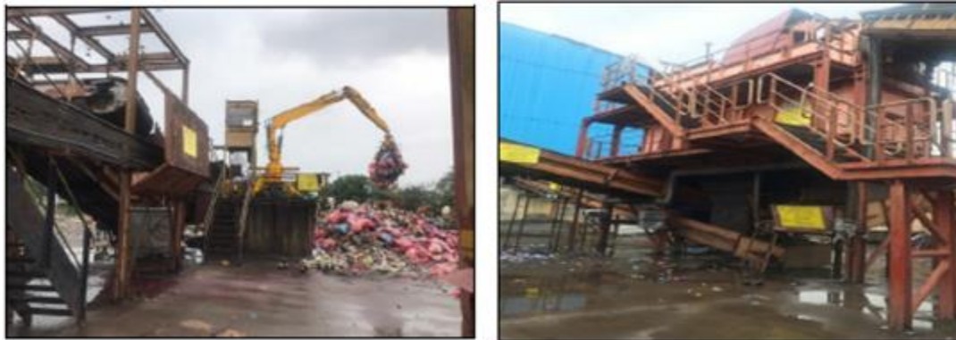
RDF plant in operation at village Langriawas, Jaipur
